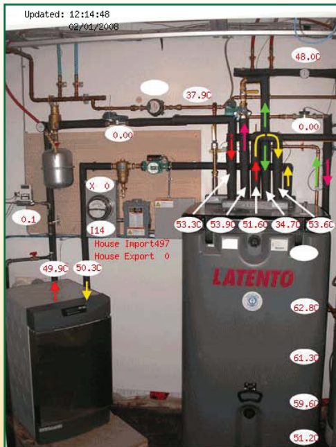
Hydronic Boiler Experiment
